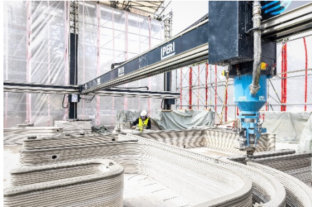
Image 1: Germany's first 3D-printed house is being built in the North Rhine-Westphalian town of Beckum. Upon completion, it will be heated, cooled and ventilated with high-efficiency solutions from Viessmann. (Image: PERI GmbH)
